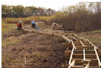
Volunteers framing the boardwalk in the Eagle Segment near Low Prairie SNA and Brady's Rocks
